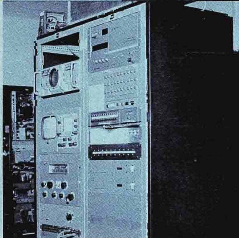
5 TT-50FH transmitter is equipped for remote operation, with a BTR-30 system (right) and automatic logging at the studio.
