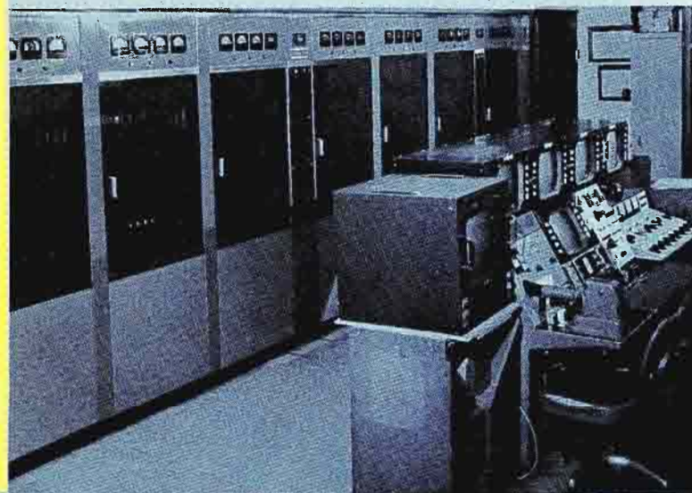
4 The durable TT-25AH 25 kW transmitter system is retired, but still housed in the KFMB transmitter building. It occupies considerably more floorspace than does the new 50 kW system.
