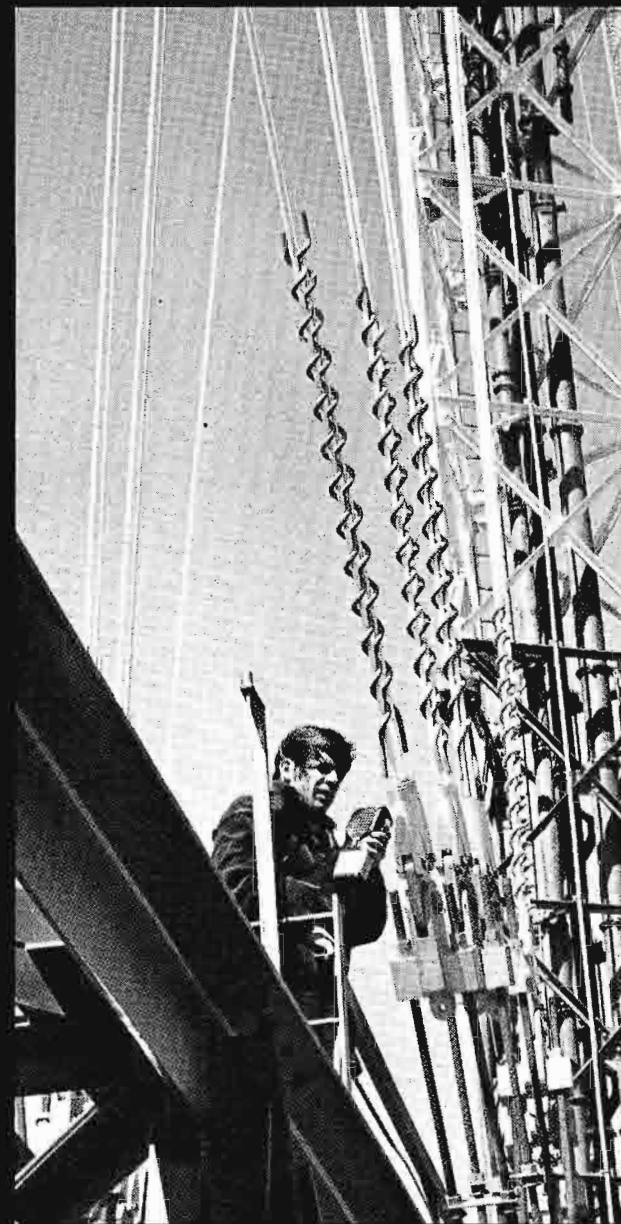
STANDBY TRANSMISSION LINE runs are contained in one tower leg; main lines in the second, and an elevator in the third.
