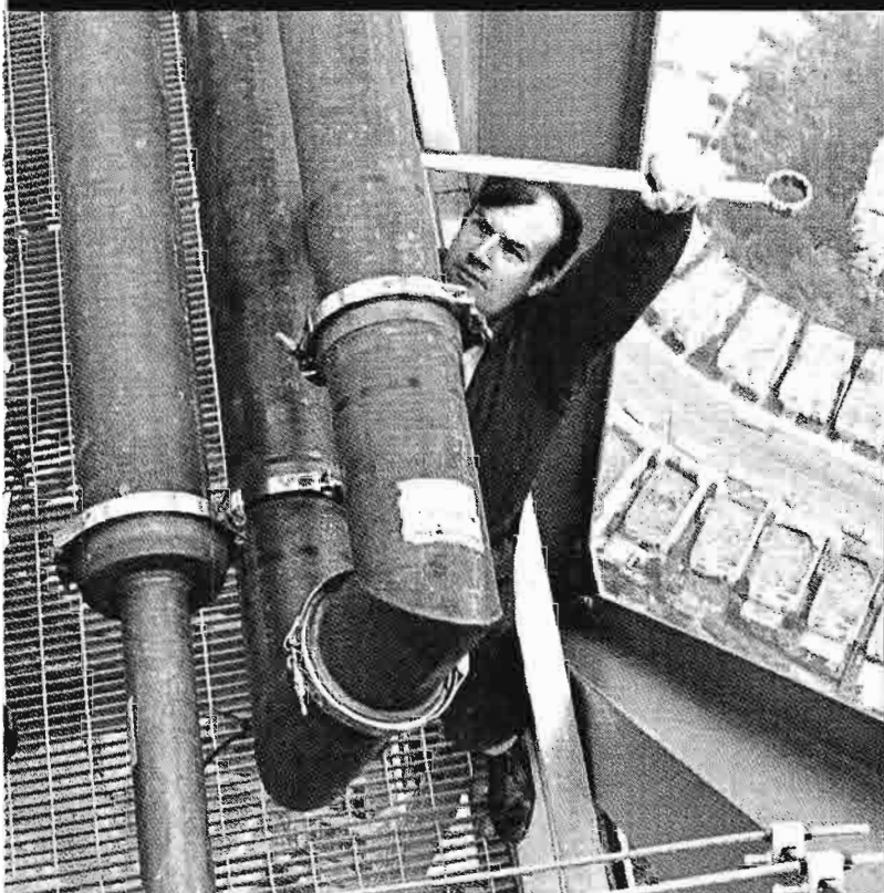
RCA ENGINEER JOHN BARBOUR tightens a connection on one of the upper lines.
